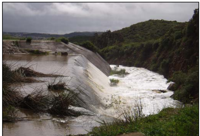
The overflow from heavy rains – February 2005
