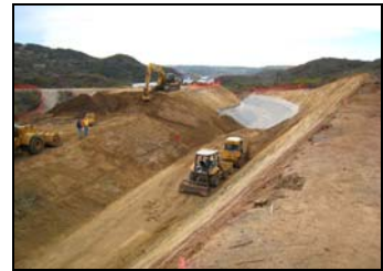
Work begins on the 'spillway' part of the Lake Calavera dam project
