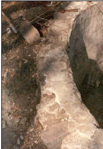
This picture shows the wall of the cistern that held rain water. The picture was taken prior to construction of the Community Center.
