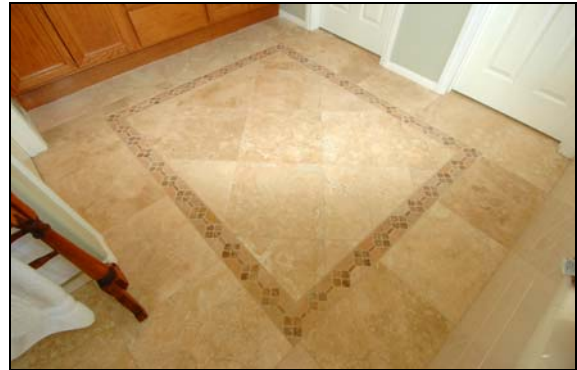
A travertine floor with an inlay, needs sealing about once per year
